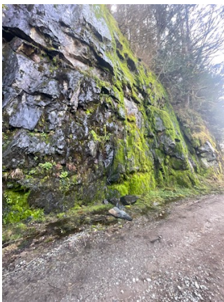
Rock fall debris
