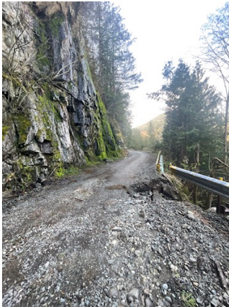
Approach from woods, erosion washout visible
